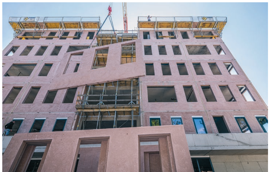
Office tower with best working atmosphere: The UNIT Tower, a seven-story office and commercial building in Gleisdorf (Styria) was realized with 2,300 square metres of precast "Ziegelit" walls as well as precast stairs and balcony slabs. Only 3 working days were required per floor!
