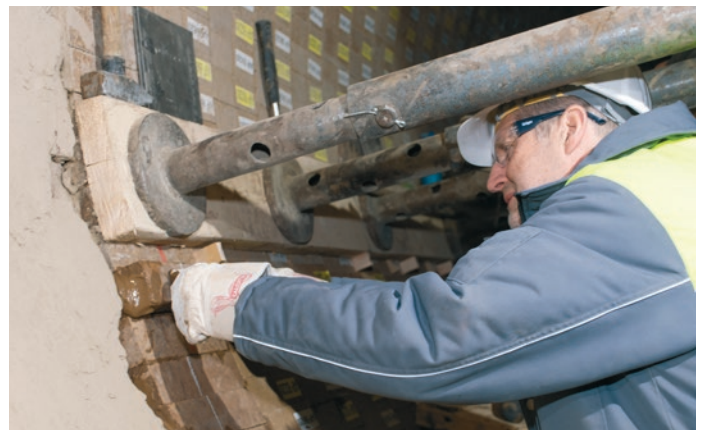
Final stone of a record-breaking repair: Plant manager Christian Breitenbaumer expertly placed the last stone.
