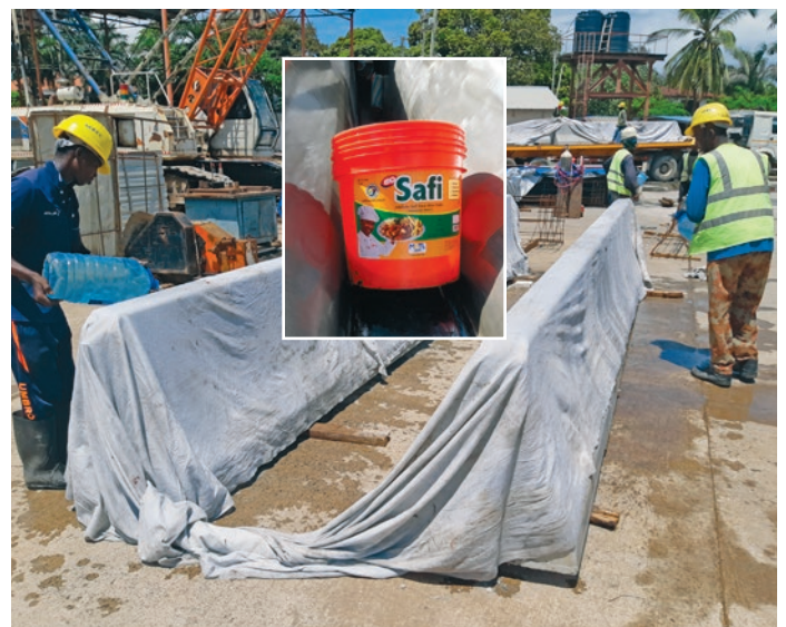
Quality by any means and tricks: Instead of mould oil, commercially available deep-frying grease had to be used. Due to the high heat, the fresh concrete barriers had to be cooled with damp sheets in order to slow down the hardening process.
