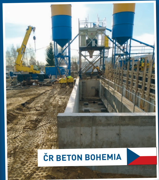
Winter construction site with speed: The comprehensive construction work as well as the technical upgrade of the ready-mixed concrete plant Strakonice could be carried out within only four months.
