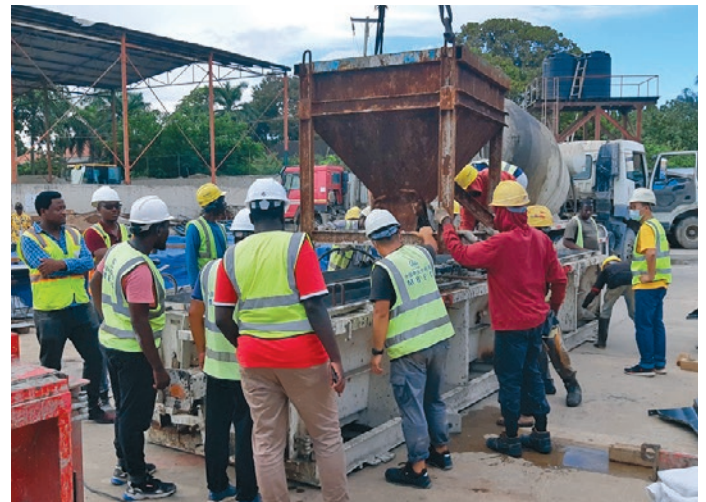
Curious employees, involved with heart and soul: There was no shortage of dedicated workers for the concreting. After the successful demoulding of the first elements, there was even dancing and singing!
