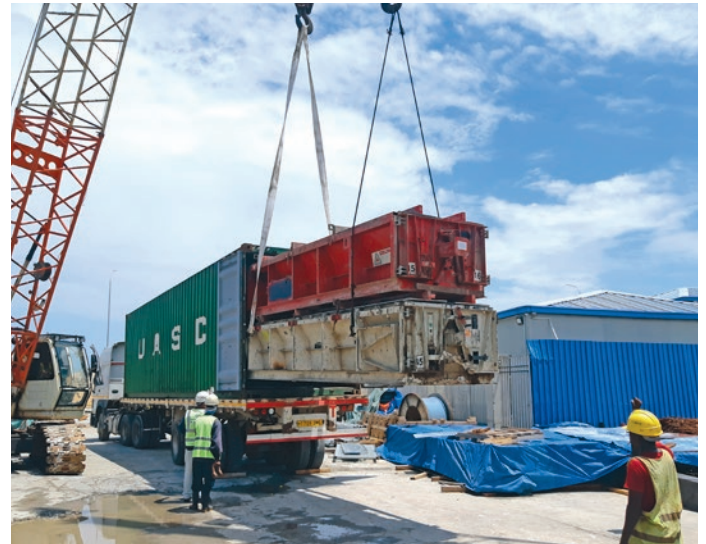
Delicate operation unloading the moulds: Without a forklift, unloading proved to be very delicate work. But the employees of the local construction company had everything under control.
